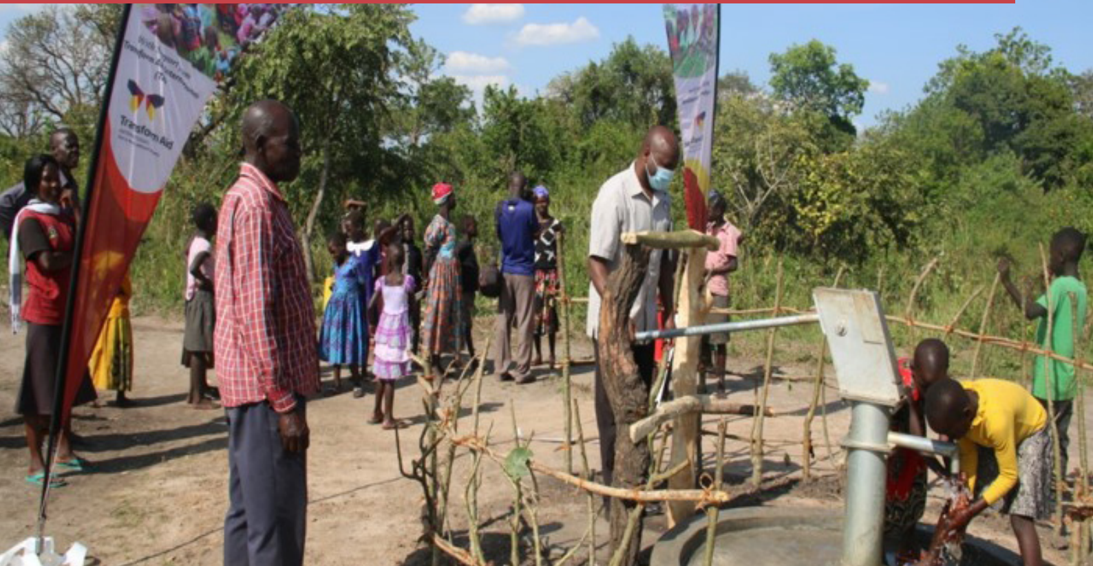
A community borehole constructed by Share An Opportunity Uganda in Kaberamaido with the aim of ensuring that communities have access to clean water.
